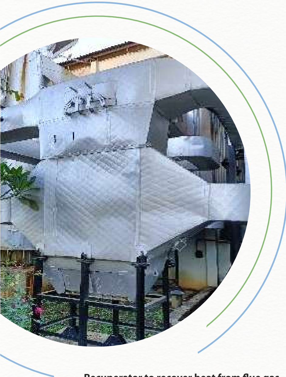
Recuperator to recover heat from flue gas to heat incoming air in ETB
